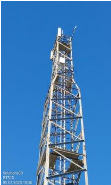
Figure 42: BTS 10 Site (Spain)
