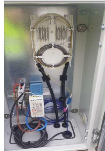
Figure 50: Internal view of the cabinet
