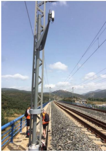
Figure 49: Trackside antenna on top the composite pole.
